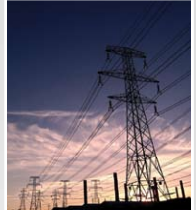
Electric utility substations Switchgear
