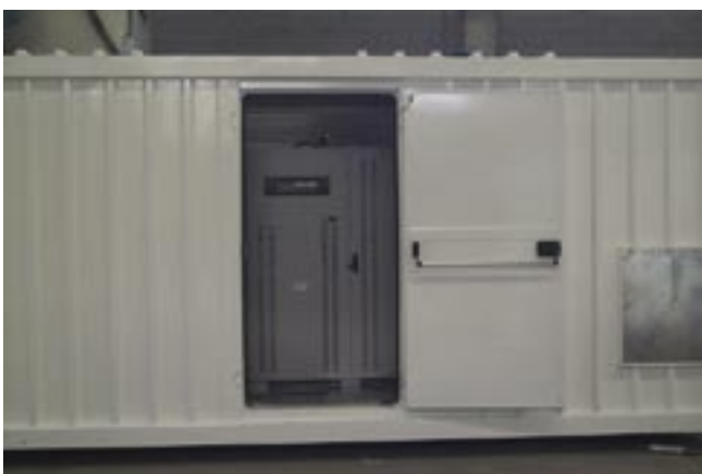
UPS mounted in a shelter
