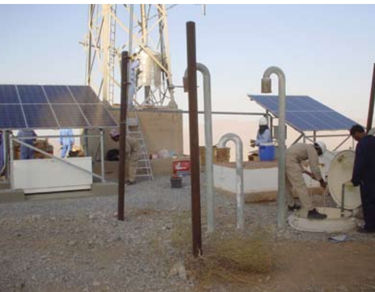
Location: Oman System Size: 1.9 kW
